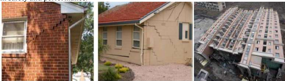
(a) Wall and façade failure (b) wall and window failure (c) building failure (Song, 2010)
